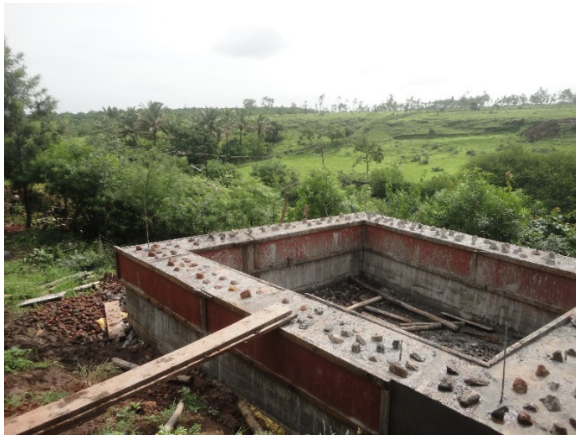
Figure 14: Rainwater Harvesting Tank
