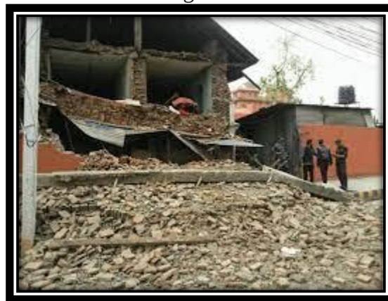
Fig. no.- 2.2 Damaged house
